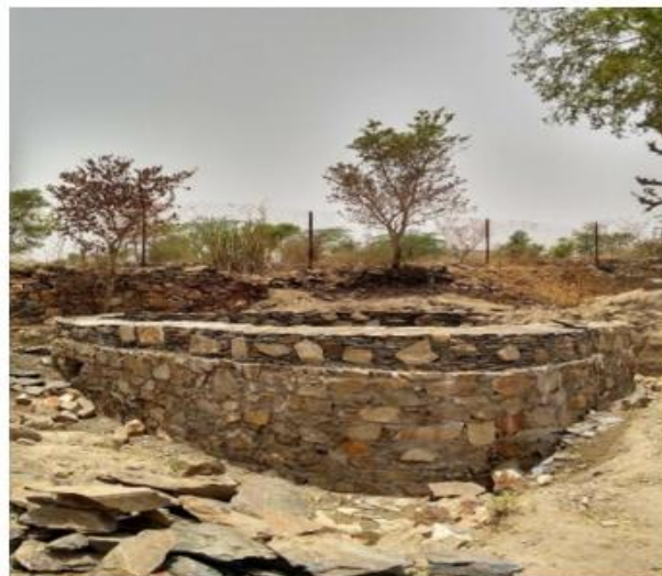
Plate 7. Open well situated at farm of Farmer C
